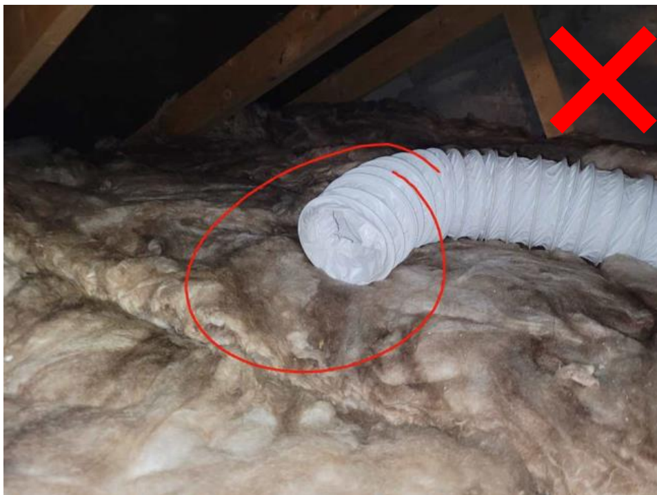
Figure 8: Example of Mechanical Extract Vent duct terminating in attic space
