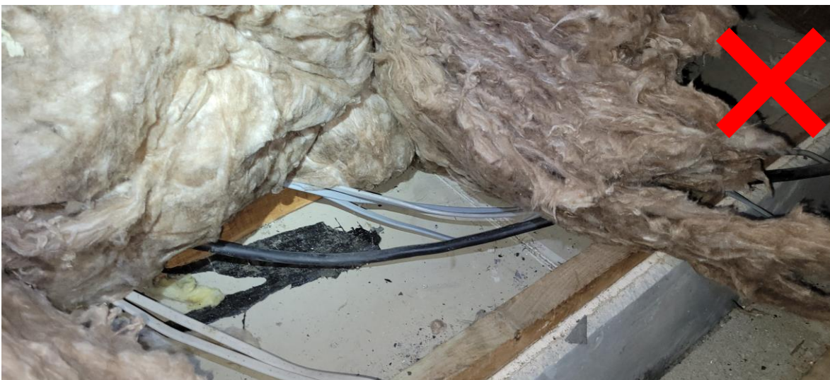
Figure 5: Example of high-powered cables being covered by Attic Insulation
