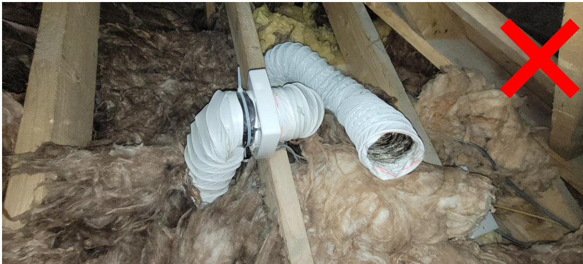
Figure 7: Example of Mechanical Extract Vent duct terminating in attic space.
